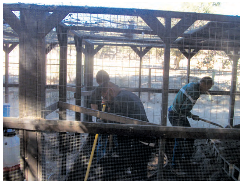
"They are digging out the dirt in the chicken coop so we can lay wire down. We got to keep the gophers out of there!"
