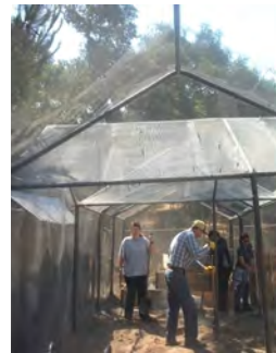
"We put the dirt inside to cover up wires around the bottom."
